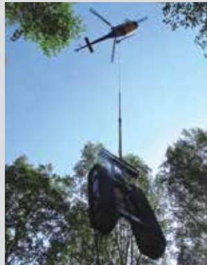
The track section of the 6712DT is lowered to a site on the mountainside to advance 4.25-in. hollow stem augers to install 2.0-in. monitoring wells.
