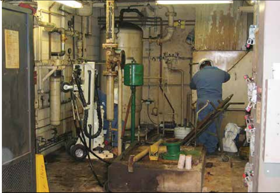
Cramped probing conditions inside building.
